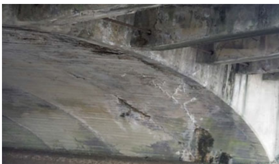
Fig. 3 Arch joint leaching and spalling
