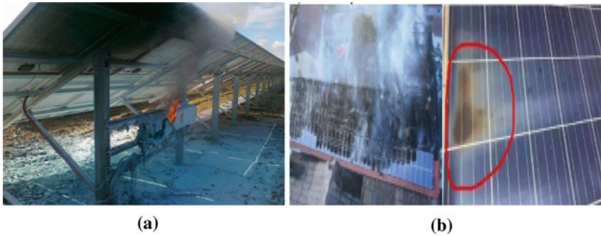
Fig. 4 a Low quality of junction box catches fire, b hotspot effect [10]
