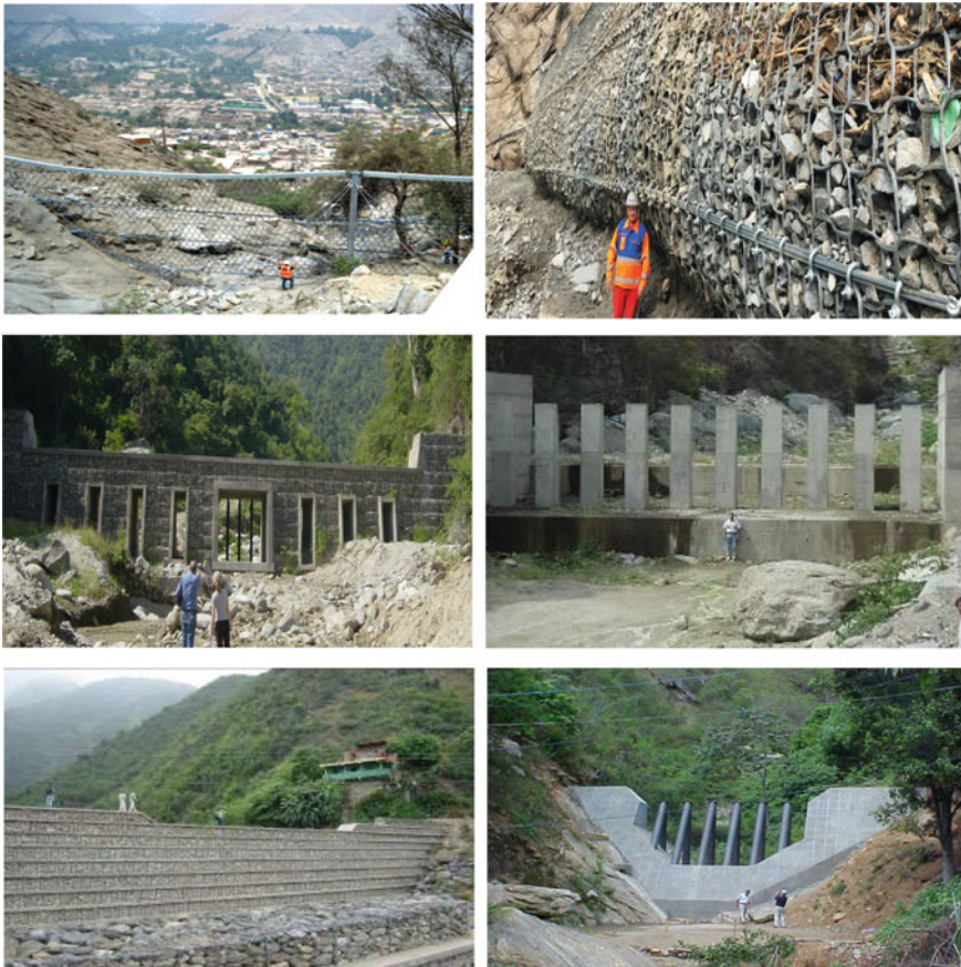
Fig. 17.8 Examples of typical torrential landslide risk mitigation works. The upper figures show metal barriers for protection against torrential landslides built in the mountains of Chosica in Lima (Peru). Source GEOBURG cited on IADB (2021c). The figures in the middle and bottom of the page show different types of mitigation works built in the watersheds of Vargas state. Source López (2011) cited on IADB (2021b)
