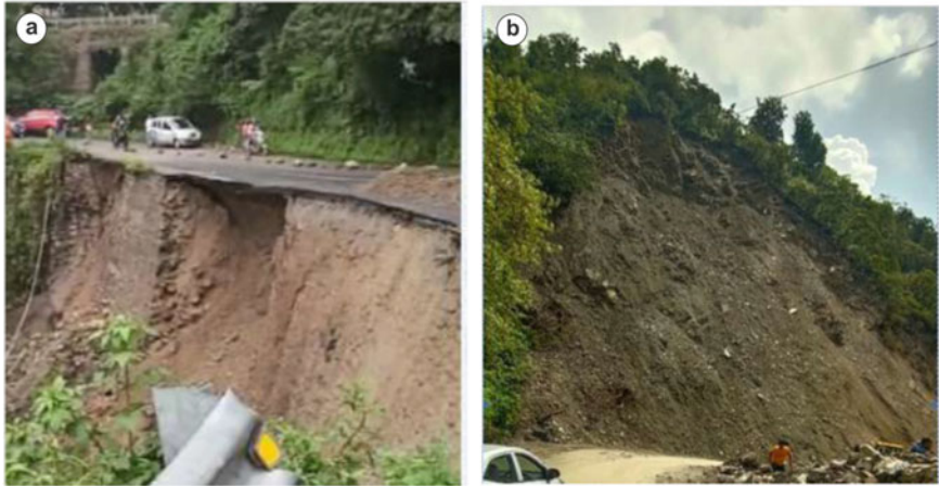
Fig. 15.5 a Damaged part of the road due to landslide; b landslide on the Dehradun—Mussoorie road after intense precipitation in August 2020
