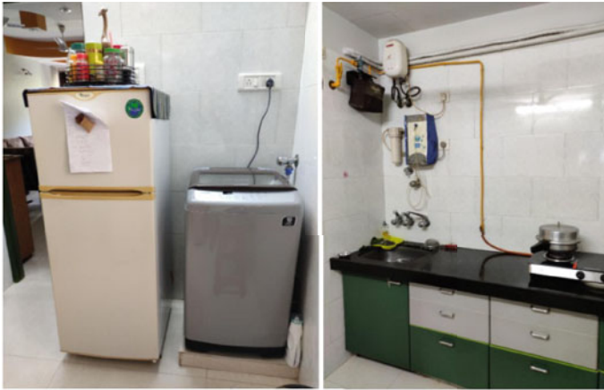
Fig. 12.1 Equipment and piping in non-industrial facilities
