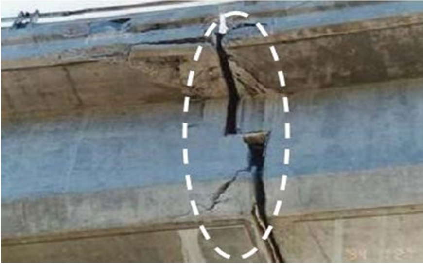
Fig. 4.10 Pounding damage in the Santa Clara River Bridge during the 1994 Northridge earthquake [19]
