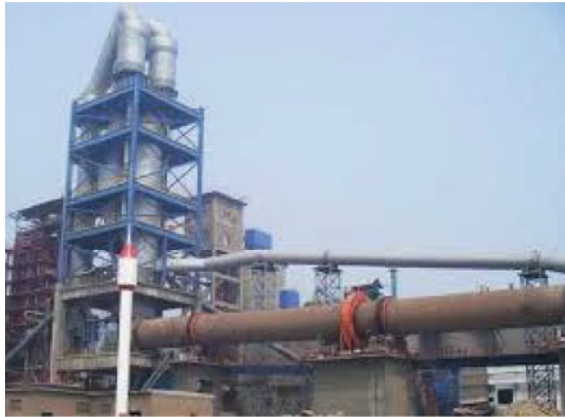
Fig. 12.2 Equipment and piping in industrial facilities
