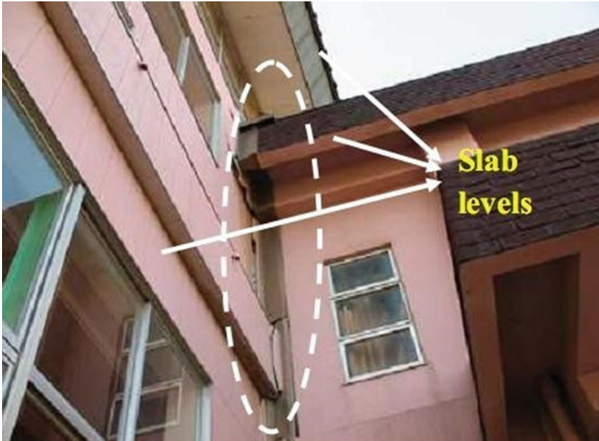
Fig. 4.12 Pounding damage due to unequal slab levels during the 2007 Niigata Chuetsu-Oki Japan earthquake [21]
