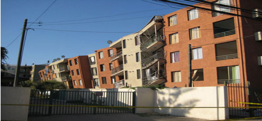
Fig. 4.6 Pounding between buildings in a row (two-sided pounding) [7]
