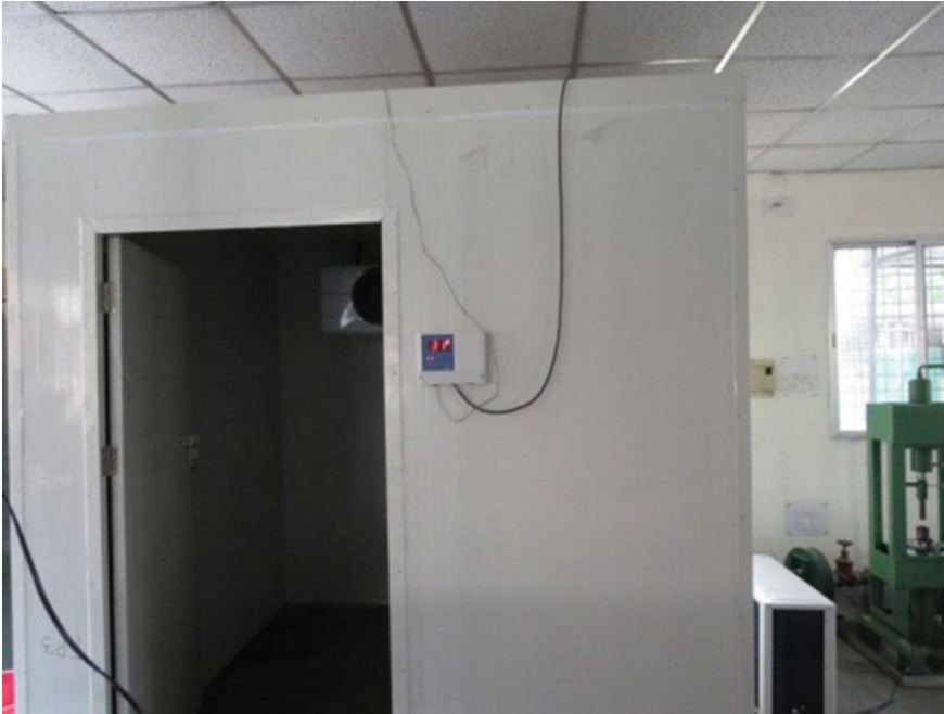
Fig. 7 Photograph of cold storage unit
