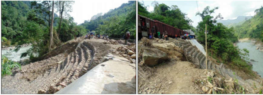
Fig. 2 Slope fails and causes sliding failure on railway embankment of Lumding-Badarpur Line
