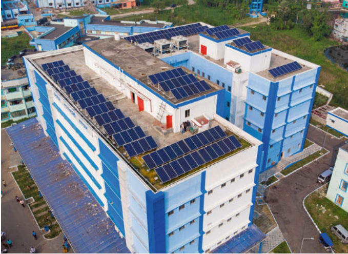
Fig. 4 Picture of the installed rooftop solar power plant
