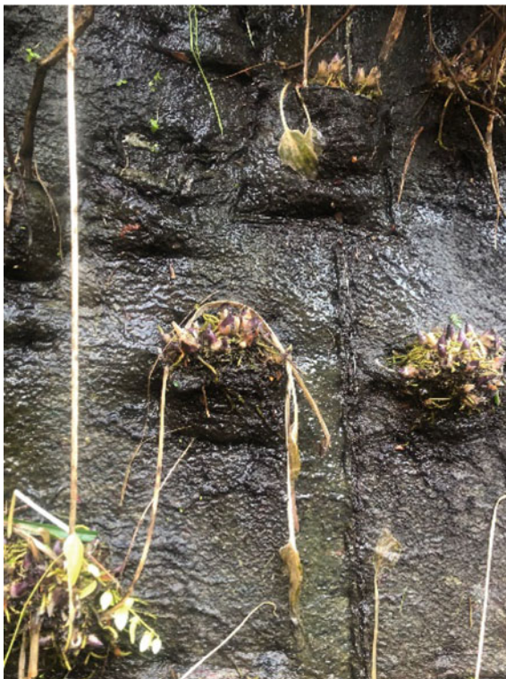
Fig. 3 Excess of the substrate moisture in the bottom parts of Caixa Forum LWS due to the insufficient drainage system. Photo by: Manouchehri. M
