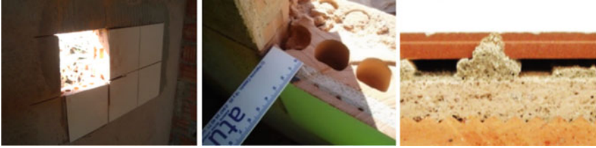
Fig. 8 Good adhesion of the mortar to the masonry and adhesive. Homogeneous distribution of the mortar on the surface of the brick
