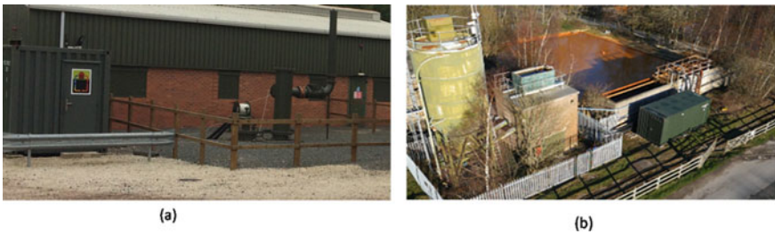
Fig. 4 Photographs of the system in Markham (a) and Caphouse (b)
