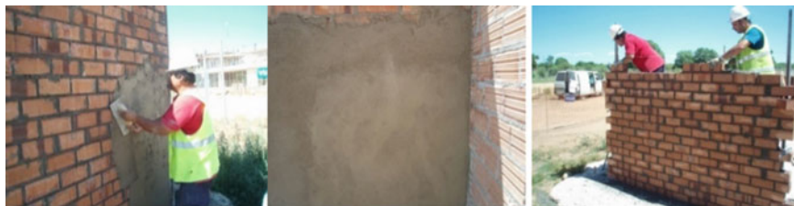
Fig. 4 Application of the plaster in the first layer and partial burnishing of the wall. Execution of the 1/2 foot wall
