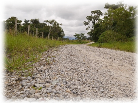
Fig. 6. Current state of the road to Morro de Calzada.
