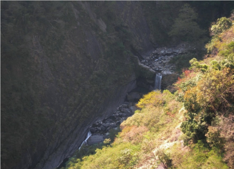
Fig. 1. Collapse of a small sediment retention dam
