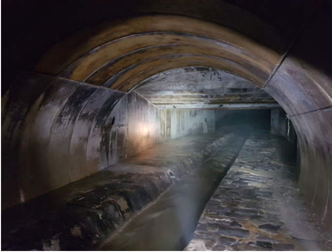
Fig. 61.2 Photograph of the inside of the Flon River vaulting looking downstream. The photo was taken at the location where the historical vaulting (characterized by the rounded ceiling, locally reconstructed with precast concrete elements as transition from the original brick section) will be replaced for the new m3. The reduced ceiling height in the background represents the modified section for the existing m2. Picture Pierre Bourqui
