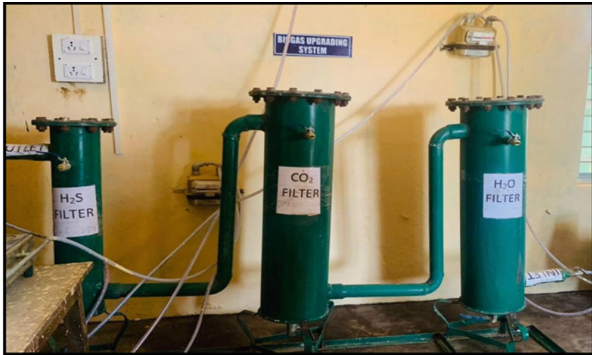
Fig. 5.3 Biogas upgrading system installed at Rewa Engineering College, Rewa, Madhya Pradesh
