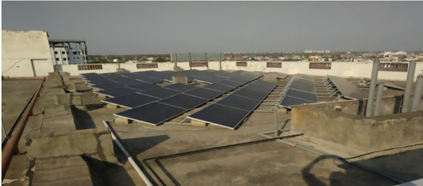
Fig. 19.7 Solar photovoltaic panels installed on Science Department Building of institute
