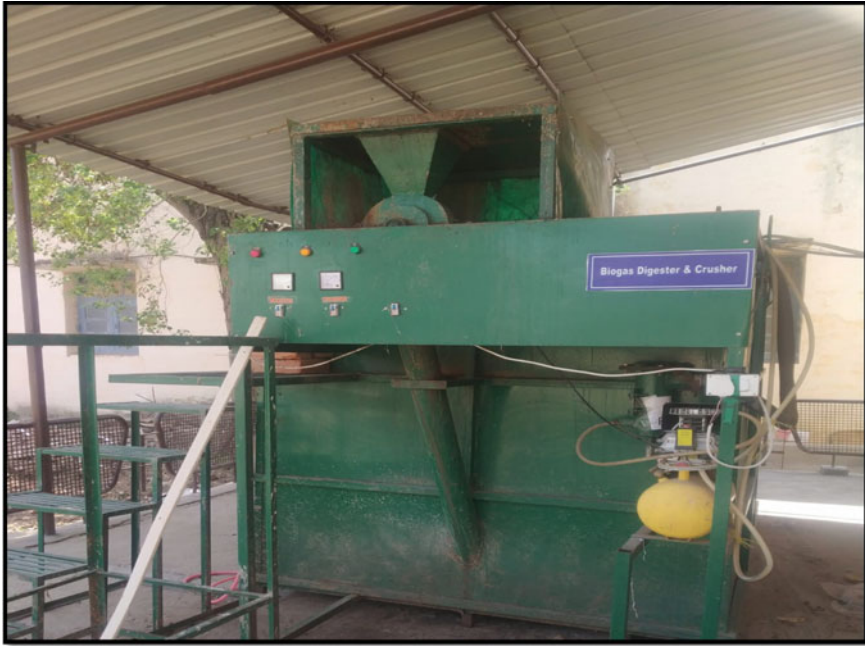
Fig. 5.2 250 kg Kitchen waste biogas digester installed at Rewa Engineering College, Rewa, Madhya Pradesh
