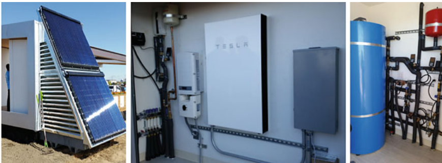
Fig. 3 Solar thermal units; Tesla storage battery; mechanical pod interior with storage tank and controls
