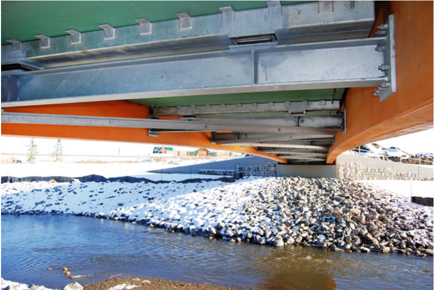
Fig. 7 Underside of bridge showing the connection between floor beams and glulam girders
