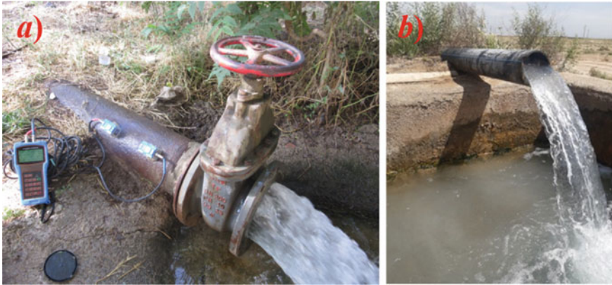
Fig. 22 Well pump outlet a full pipe flow, b partially filled pipe flow
