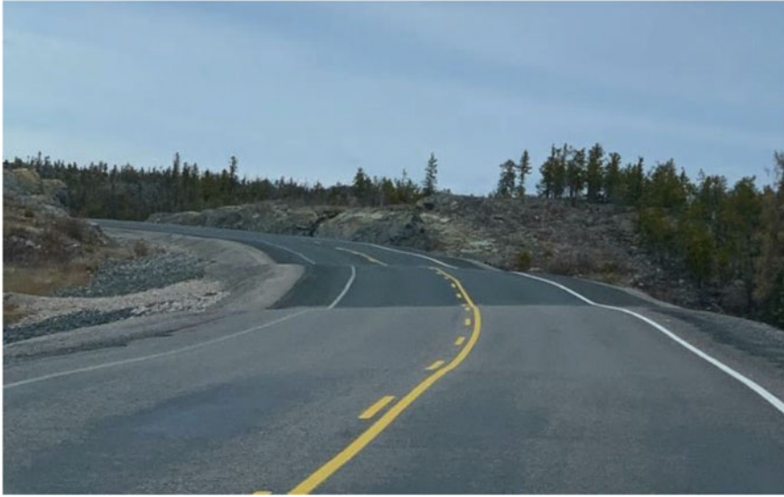
Fig. 1 Differential Settlements of the road structure along Ingraham Trail [13]
