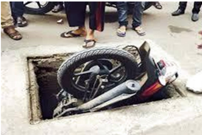
Fig. 1 Accident due to missing manhole covers [2]
