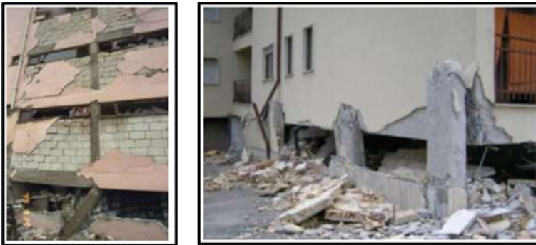
Fig. 6 Column failure and building collapse
