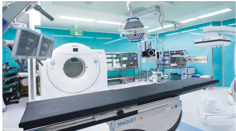
Fig. 23.3 The hybrid operating room is equipped with a 3D robotic C-arm (the Artis pheno by Siemen Healthineers), a CT scanner, and a navigation system
