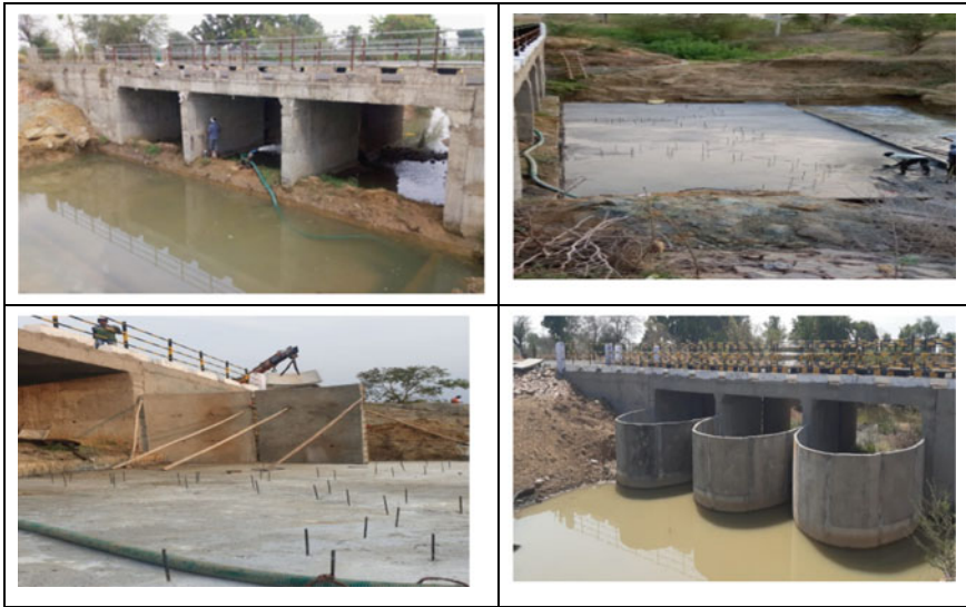
Fig. 6 Elliptical arch wit standing water and back water also shows construction technology
