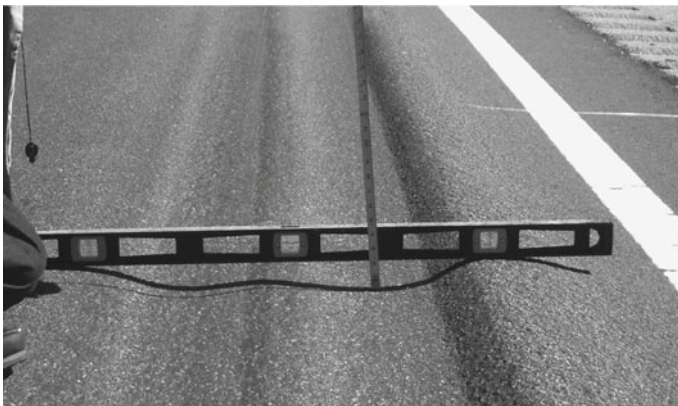
Fig. 8 Rut failure in bituminous layer. Source MS 2 2014
