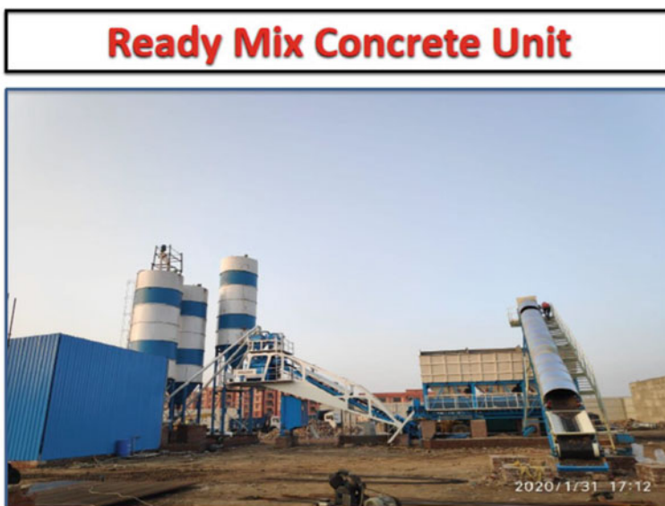
Fig. 6 Photograph showing Ready Mixed Concrete Unit
