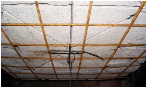
Fig. 41 Concrete sections on the top of the steel mesh (after Nemcik et al. [18])
