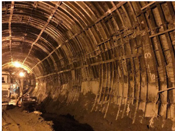
Fig. 23 Stage wise benching in critical reach and extension of ribs from springing level
