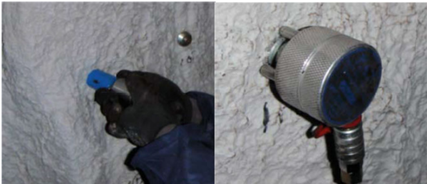
Fig. 39 In situ adhesion strength test showing overcoring on the left and dolly under test on the right
