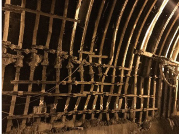
Fig. 19 Twisted and misaligned ribs at RD 998 m (0.62 miles)
