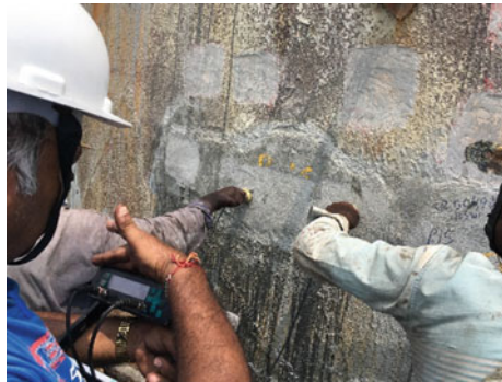
Fig. 19.9 UPV testing over polymer modified mortar used in repair of RCC chimney by surface probing method
