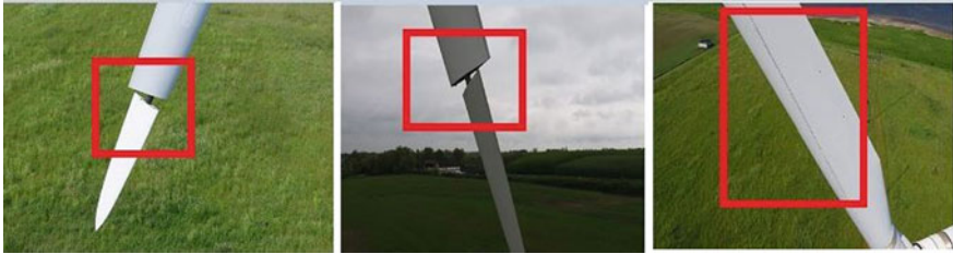
Fig. 1 Breakage and surface defect [6]
