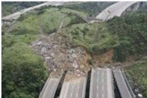
Fig. 1 Photograph of freeway No. 3 landslides in Taiwan [3]
