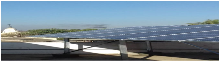
Fig. 1 Plant site view
