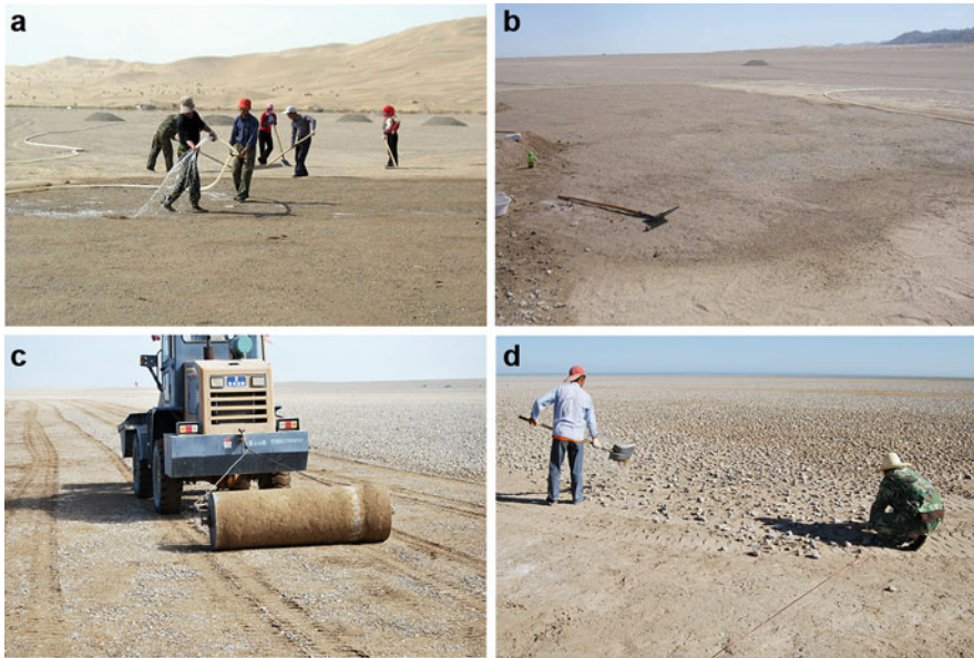
Fig. 10.12 Process of paving gravel on the sandy gobi, including watering (a), paving mixed soil (b), rolling (c), and paving gravel (d) (provided by WM Zhang)
