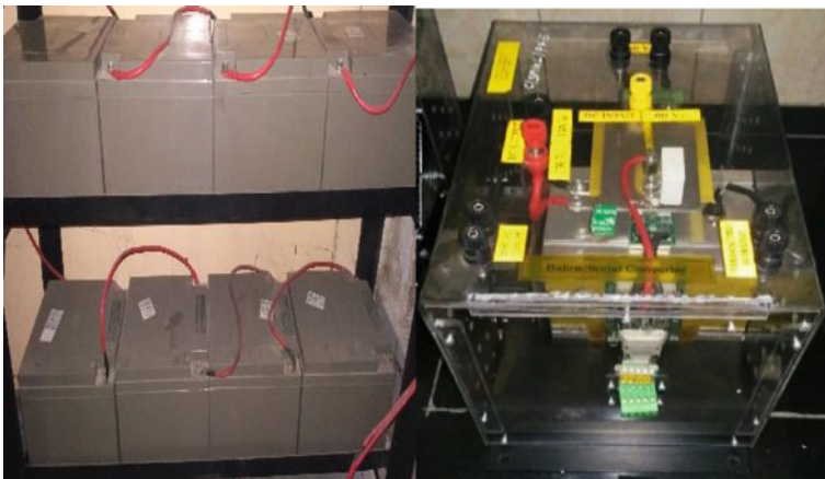
Fig. 6 Battery bank with bidirectional converter
