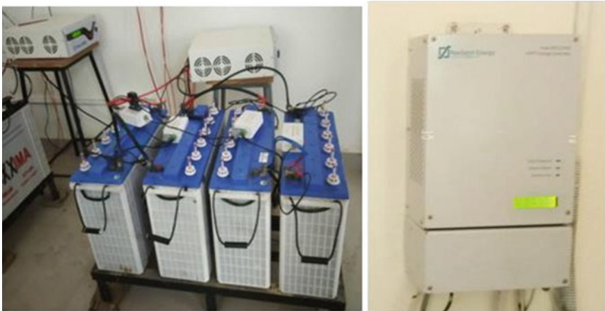
Fig. 4 Battery Storage System and MPPT System with Charge Controller
