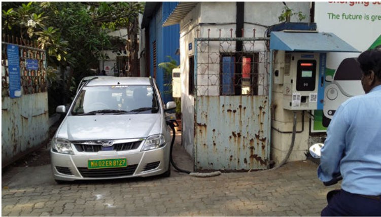
Fig. 5 Fleet vehicle is being charged at 10 kW DC charging station in KalaNagar BKC
