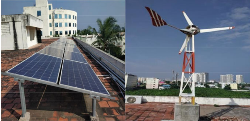
Fig. 3 Solar Panel 5KW installed in the Campus and 1KW Wind Mill PMSG installed
