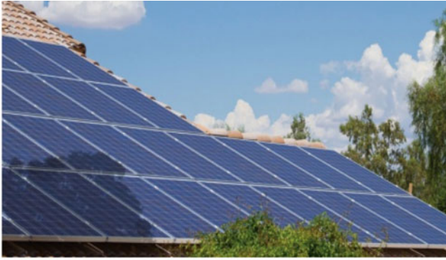
(a) Real PV System
