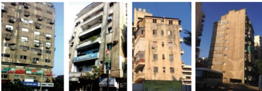
Fig. 1 Example of exterior stained façade in Cairo, Egypt
