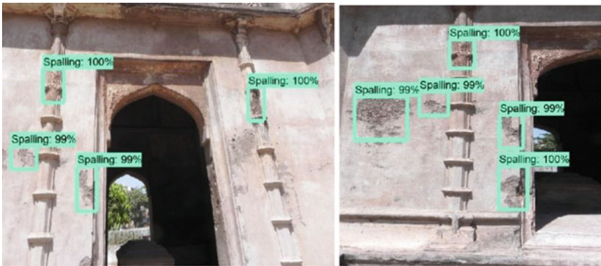
Fig. 6 Detected defects— spalling
