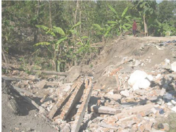
Fig. 7 The damaged house built on unstable ground [18]
