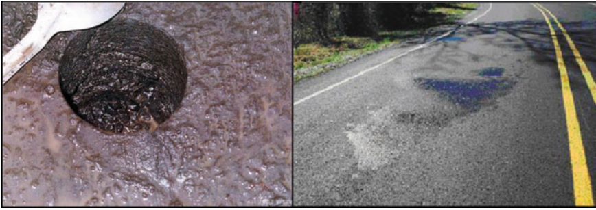
Fig. 3 Stripping occurs in the surface and subsurface pavement structure
