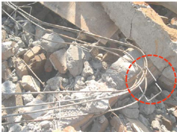
Fig. 5 Brick masonry with poor detailing of stirrup reinforcement [18]
