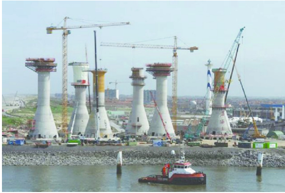
Fig. 2. Assembly line for fabrication of offshore wind turbine foundations for Thornton Bank, Belgium [7].
