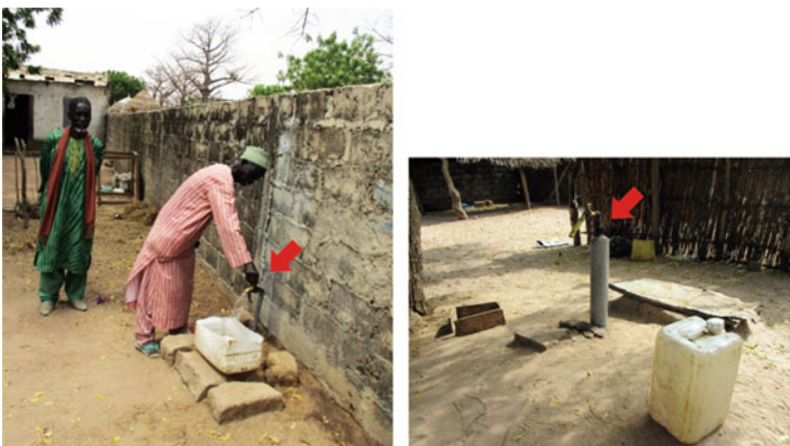
Fig. 4.4 Water supply faucet installed in a household of rural villages in Senegal (the left photo was taken in the Fissel Deux village chief's yard, and the right photo was taken in the Mboudaye village chief's yard). (Photos by Ikemi)
