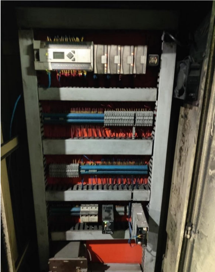
Fig. 5 PLC panel with required protection
