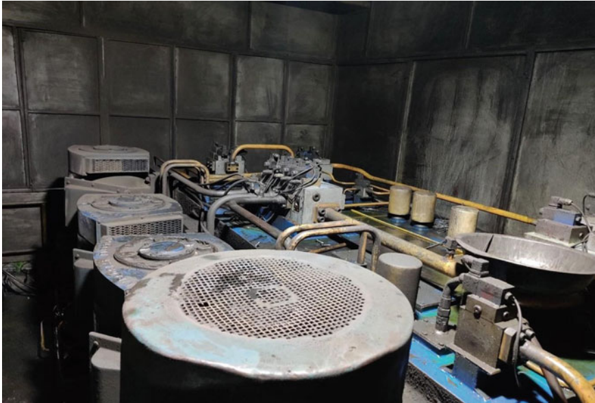
Fig. 6 Added metallic box-like structure with blower fan to maintain temperature
