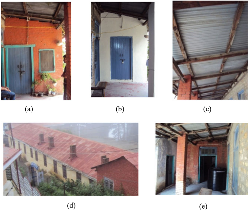
Fig. 20 a, b Store room window to be removed, c Corridor roof, d Chimneys to be removed, e Corridor roof subjected to leakage
