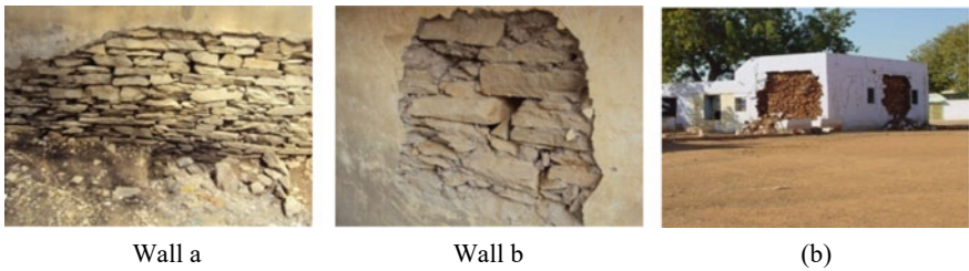
Fig. 11 Random rubble masonry wall a Shimla school b Damaged during Bhuj earthquake
