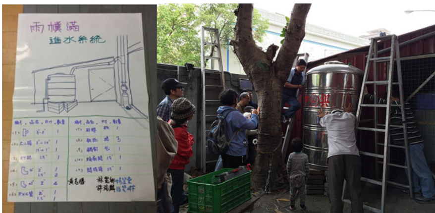
Fig. 22.2 Design diagram for a rain-harvesting system (left) and volunteers installing the system in a local junior high school on March 21, 2015 (right)
