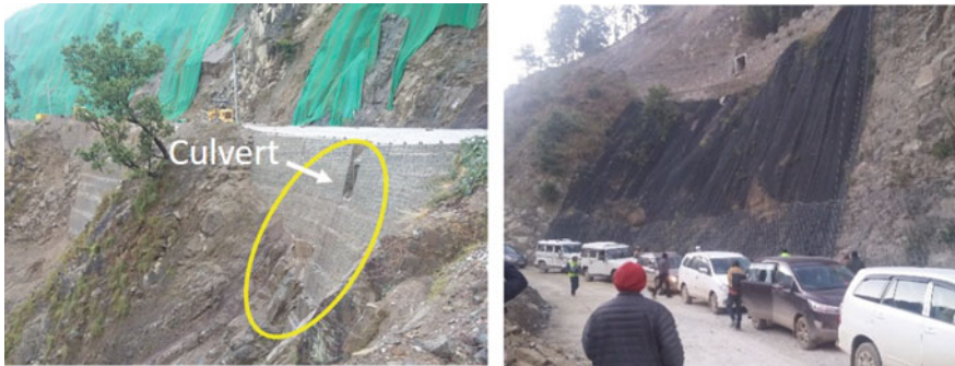
Photograph 9 Culverts left open without stepped chutes on downhill slope
