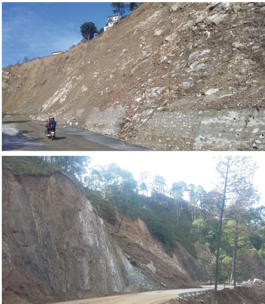
Photograph 6 Landslides are created due to steep cut slope
