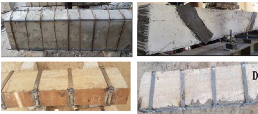
Fig. 1 Various techniques for retrofitting beams employing threaded bars and welded steel plates [1]
