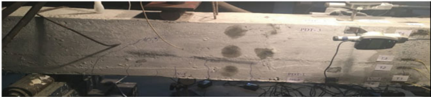
b) Cracks in experimental beam, with the below layer of steel fiber concrete
