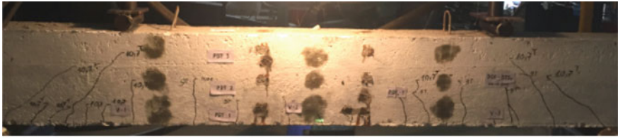
a) Cracks in experimental beam, with the above layer of steel fiber concrete
