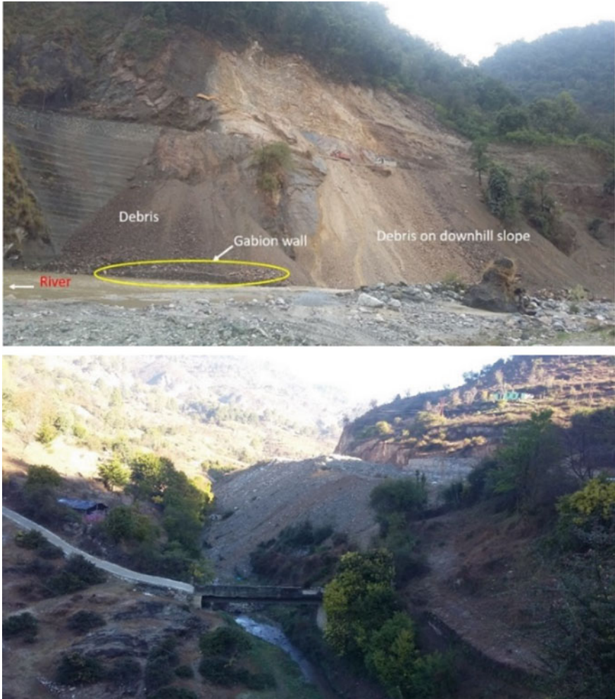
Photograph 8 Dumping of excavated material on a downhill slope in river portion
