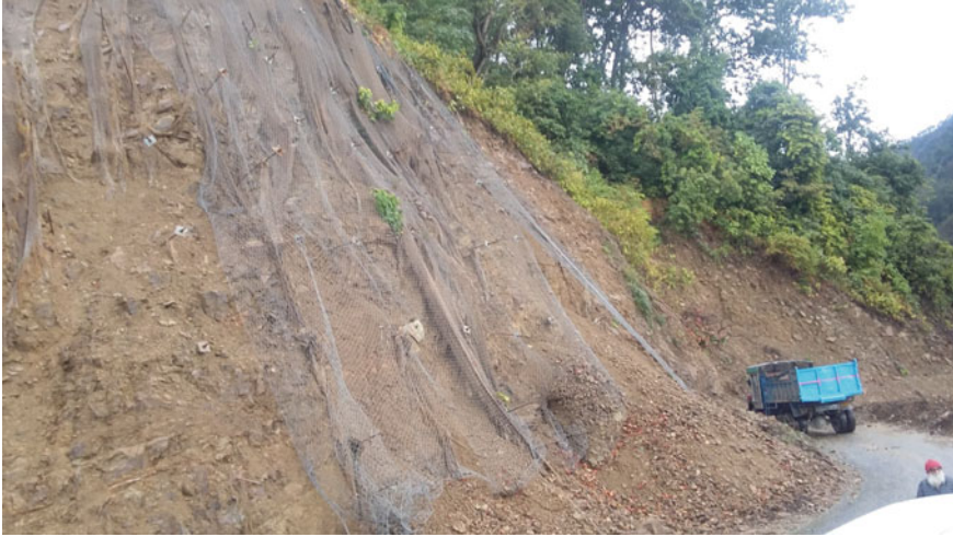
Photograph 4 Slope protection measures are implemented. But, failed due to activation of slide
