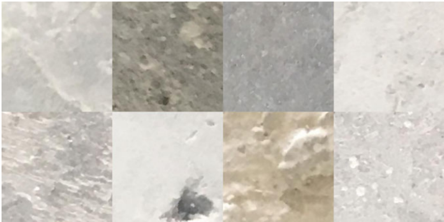
Fig. 3 Sample concrete surface images with no-crack
