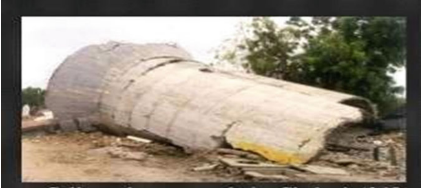
Fig. 1 Failure of water tank
