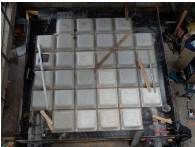
Fig. 1 General view of the formwork under the slab before installing the reinforcement cages
