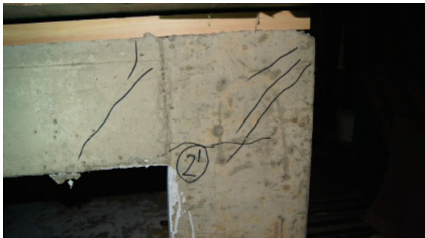
Fig. 6 The nature of cracks on supports at a load of 10 \text{ kN/m}^2
