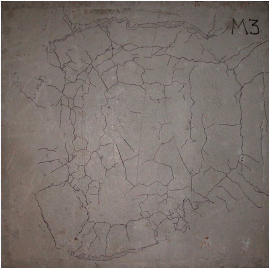
Fig. 3 Prototype in [7] after punching failure. Tensioned surface
