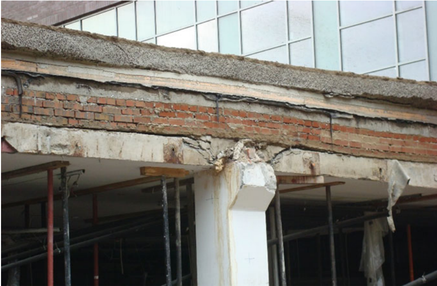
Fig. 4 Flat slab after punching failure
