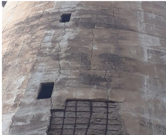
Fig. 2 Completely deteriorated side of the tank
