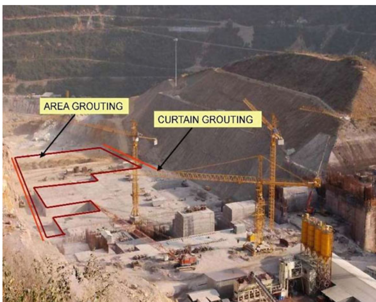
Fig. 10 Location of consolidation/ area grouting and curtain grouting in terrace material portion
