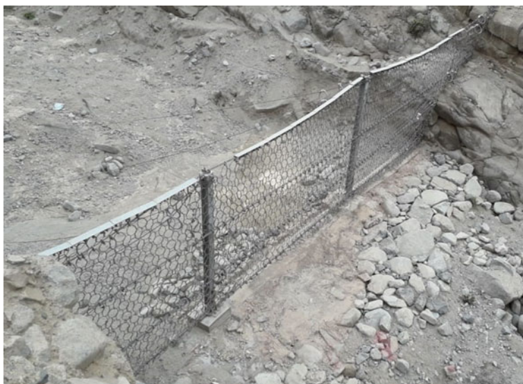
Fig. 2 Flexible debris flow barrier of the Quirio creek
