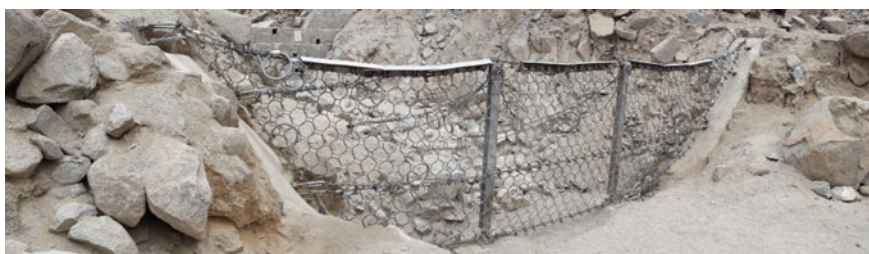
Fig. 4 Flexible barrier of the Castilla creek
