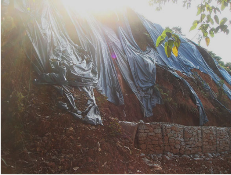
Fig. 3 Landslide detected on the slope at Location B (February 2009)
