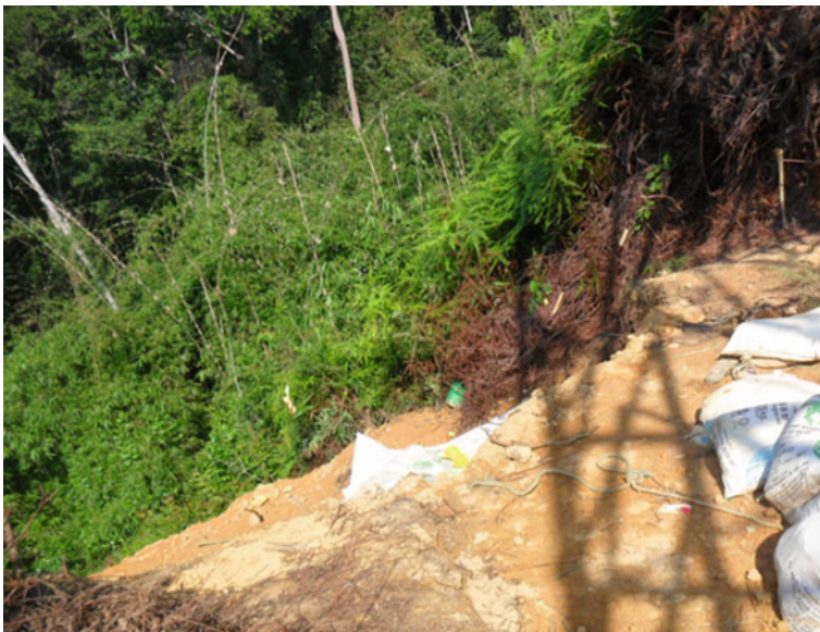
Fig. 2 Landslide detected on the slope at Location A (June 2011)
