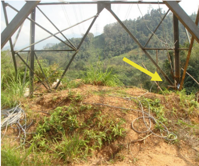
Fig. 5 Position of critical leg at Location B
