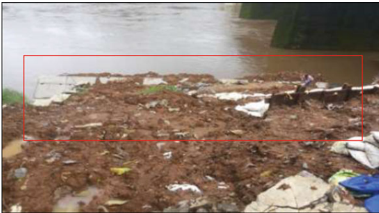
Fig. 2 Collapsed retaining wall
