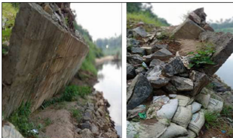
Fig. 4 Laterally displaced retaining wall
