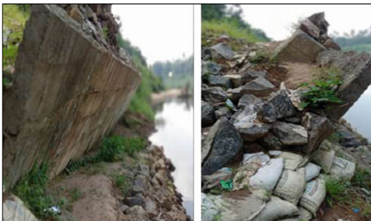
Fig. 4 Laterally displaced retaining wall
