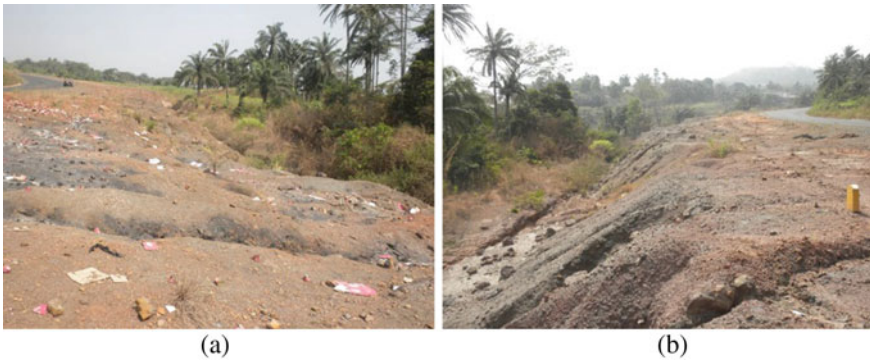
Fig. 5 Side-cast construction. a Erosion at unprotected verge. b Gullying at unprotected side-cast slope
