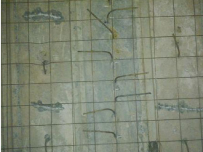
Fig. 12 Install steel on the inside of the piles wall and pour a layer of concrete 15 cm waterproofing
