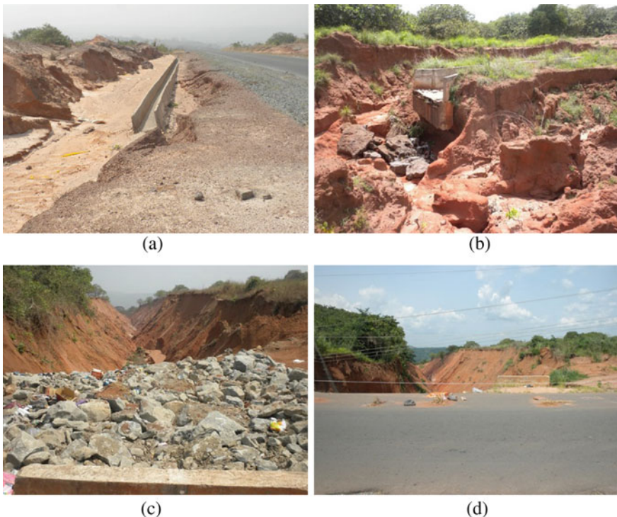
Fig. 2 a An instance of a poorly located drainage. b Gullying around culvert outlet at Km 7.0. c Gullying around culvert outlet at Km 8.6—armor protection still present. d Gullying around culvert outlet at Km 8.6—highway breached by gully
