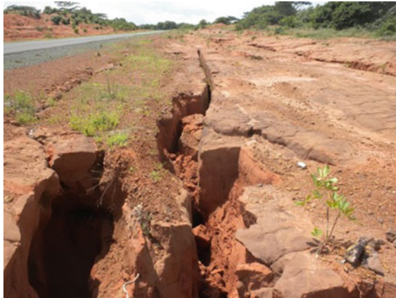
Fig. 3 Gully development from poorly reinstated utility (optical fiber) excavation
