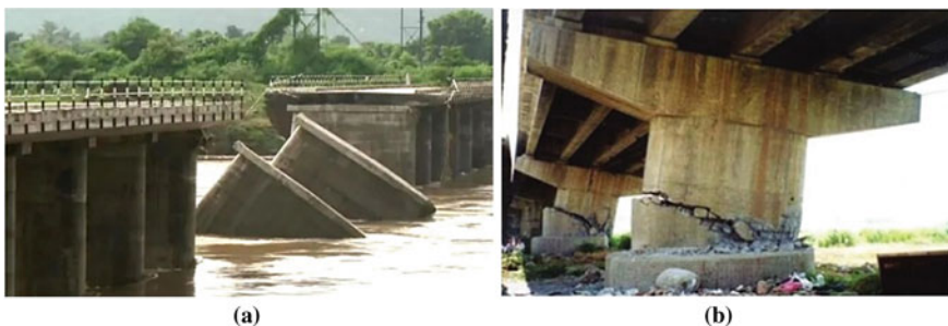
Fig. 1 Bridge collapse, a Pier failure in Ramtek, b Shear failure of pier wall (Courtesy www.ndtv.com ) (Courtesy Sung, 2009 [33])
