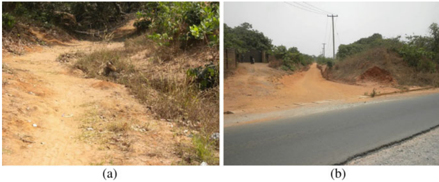
Fig. 6 a Footpath as runoff channel. b Earth road as runoff channel
