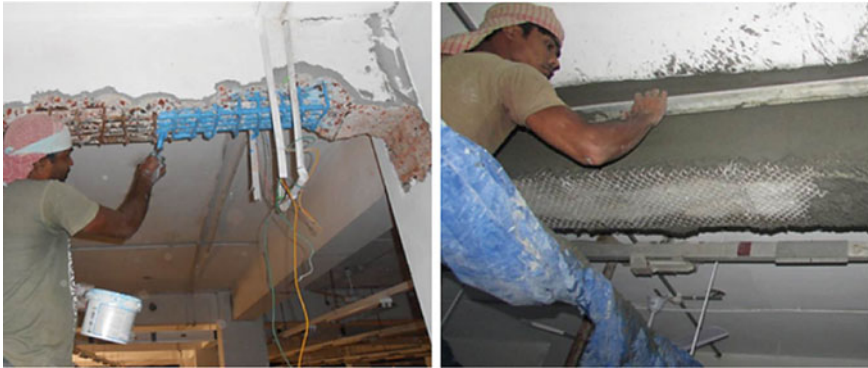
Fig. 24.3 Applying corrosion inhibitor on bottom beam rebars (left), ferro-cementing with wire mesh on beam bottom (right)
