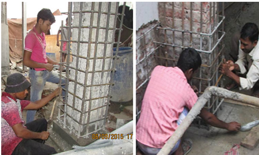
Fig. 24.2 Reinforcement placement for concrete jacketing of RCC column (left) and brick column (right) of an RMG factory building
