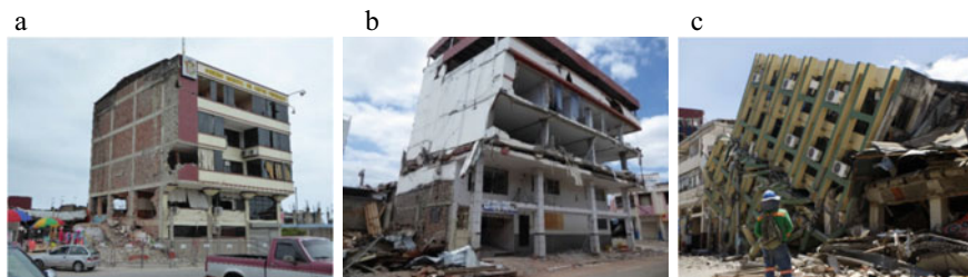
Fig. 14.6 Performance of buildings affected by the Muisne earthquake. a RC frame with masonry infill building at Pedernales, b RC building at Manta, c RC building at Portoviejo
