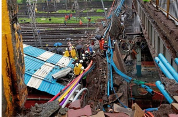
Fig. 25.2 Failure of bridge crossing the railway lines
