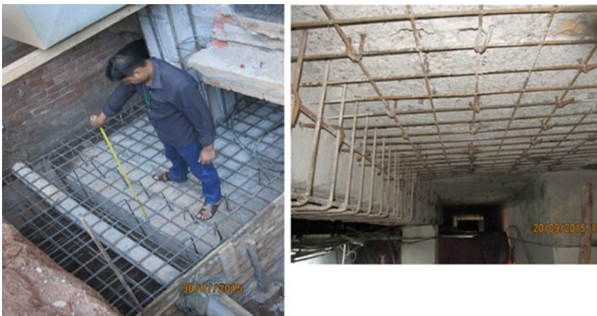
Fig. 24.4 Reinforcement placement for strengthening of RCC footing (left) and RCC slab/beam (right)
