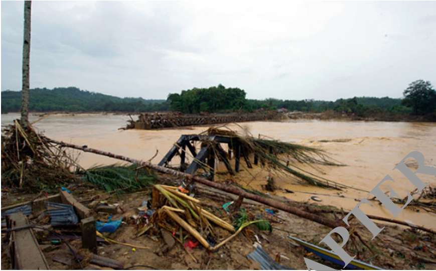
Fig. 19.3 Washway of railway tracks occurred in Malaysia East Coast Line railway bridge, which cross Nenggiri River in Kemubu, Kelantan, had totally lost due to massive flood in December 2014 (Courtesy Malaysian Department of Public Works)
