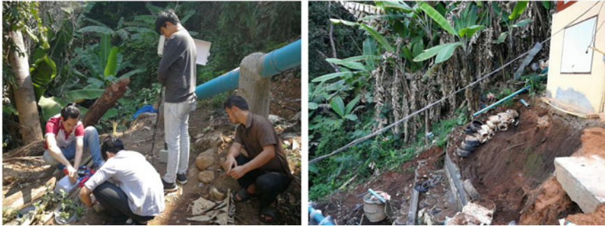
Fig. 12.2 Network installation (left) and experimental site in Chiang Mai province, Thailand (right)
