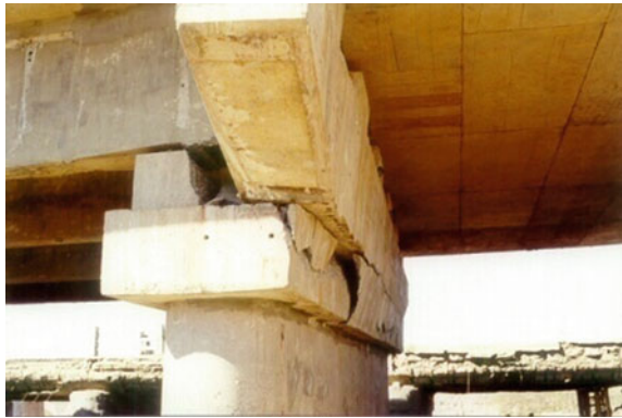
Fig. 25.5 Sliding of bridge deck and failure of pier cap during Bhuj earthquake
