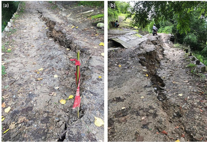
Fig. 11.11 Cracks developed in road near Pyarienii jhora during 2020 monsoon. a On 27 July 2020, and b on 6 August 2020 [38]
