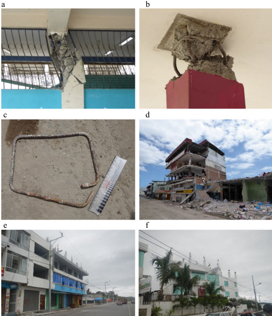
Fig. 14.9 Failures caused by inadequate design of infills and reinforcement detailing following the Muisne earthquake. a School building with short column failure, b column head failure showing insufficient shear design, c insufficient lapping of column link with no 135°-bend, d inadequate design/detailing of RC frame and infills at Portoviejo, e , f exposed reinforcement for future building extension in Ecuador.
