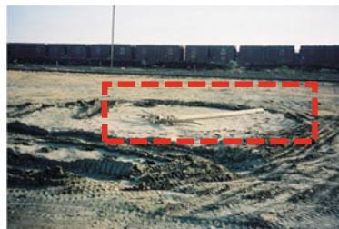
c The collapse of telephone poll due to loss of strength in the supporting soil.
