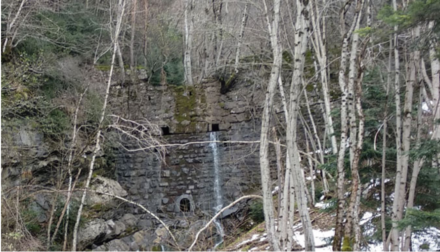
Fig. 28.5 Current state reveals the aging of the transversal dikes in San Epifanio torrent
